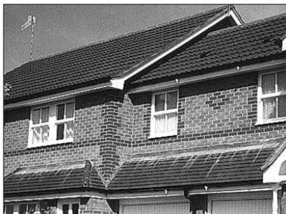
Roof tiles spoiled by run-off staining.
